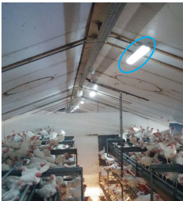
Figure 2.1-B The HD ionization lamps in the shed where the measurements were taken. In the photo, one ionization lamp is circled in blue.
